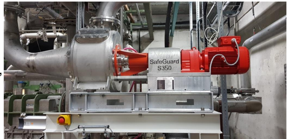
Installation in paper mill
